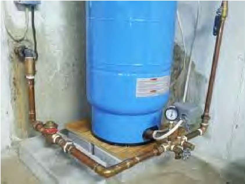
Image of how a well connects to a pressure tank, showing the pressure gauge, pressure switch and storage tank
