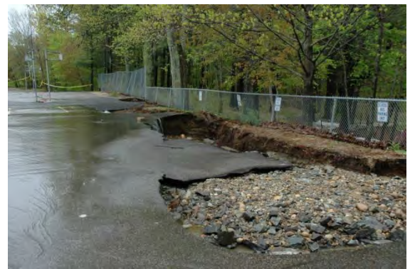
Roadway Damage from Flooding Photo Credit: Town of Newmarket
