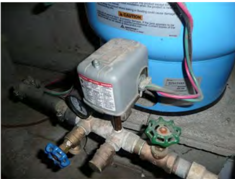
Close-up view of the pressure switch that turns the pump on/off; The blue tank is the pressure tank
