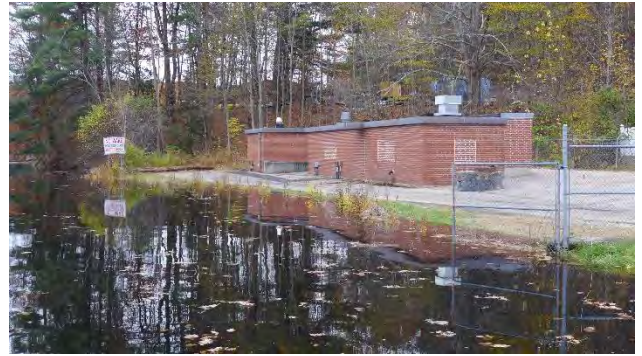
King Tide flooding at pump station on Creighton St. Photo Credit: Kyle Pimental
