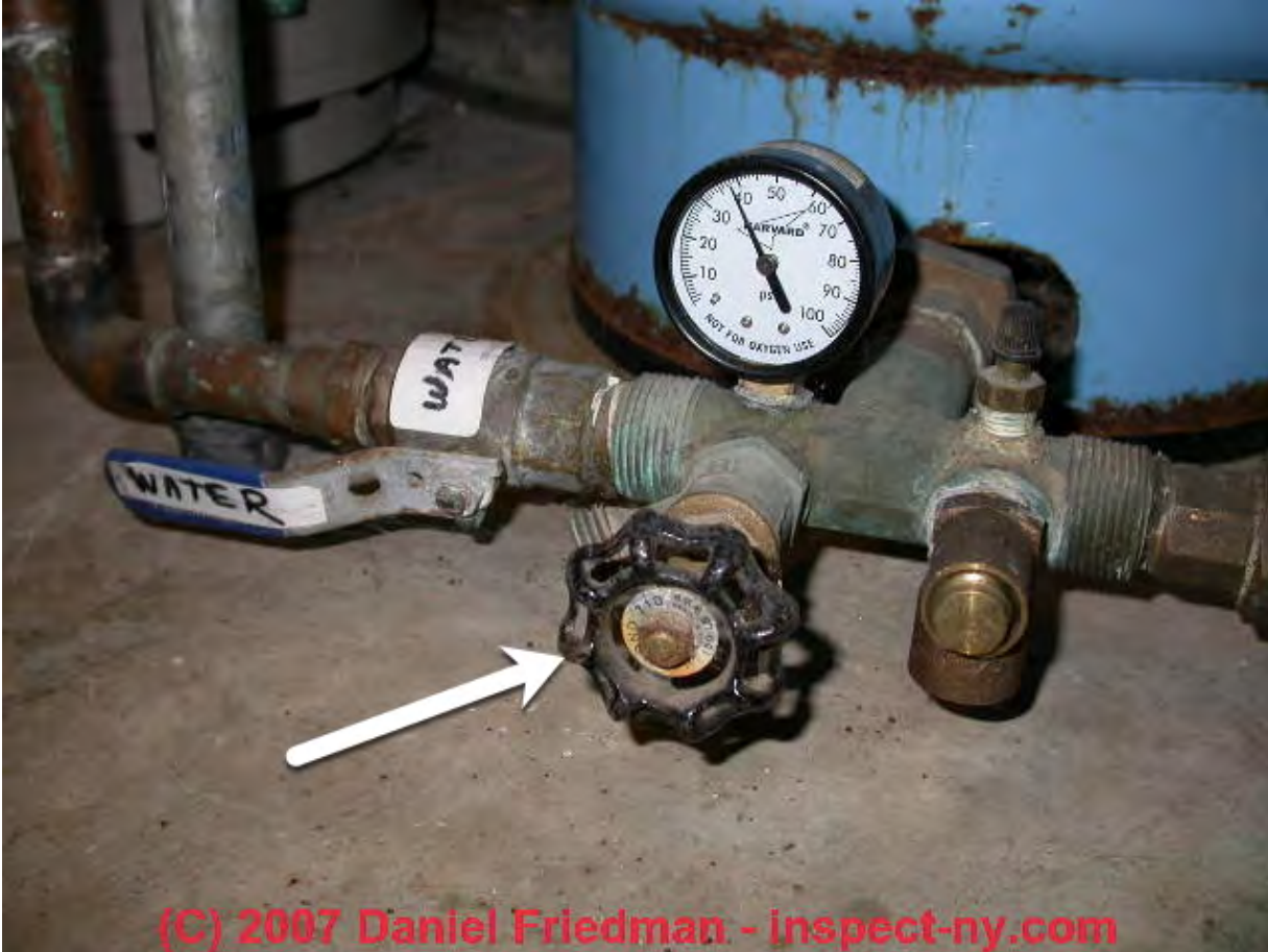
A main water shutoff valve , in this case the blue lever labeled "WATER" with white tape, is shown to the left of the pressure gauge and pressure tank drain valve in our photograph (white arrow).
