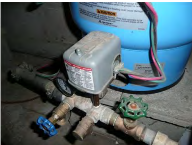
Close-up view of the pressure switch that turns the pump on/off; The blue tank is the pressure tank
